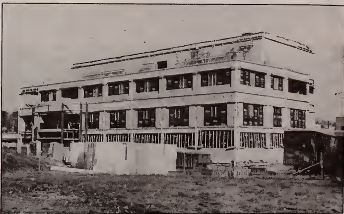
University Park construction ... The ARL Building is under construction on the West Campus at University Park. The $10 million applied research laboratory is being funded by a grant from the U.S. Navy. Projects to be housed in the three-story, 71,000-square-foot structure include studies of marine composite materials, turbomachinery and instructional fluid dynamics, ocean acoustics and active vibration control. The building also will include a 290-seat auditorium, conference rooms, a student study area, classroom space and a library.
